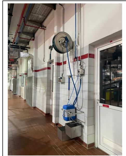
Hose reels were used to apply foams to the air conveyor rails, with hoses spanning across the hall to reach the respective air conveyor rails
